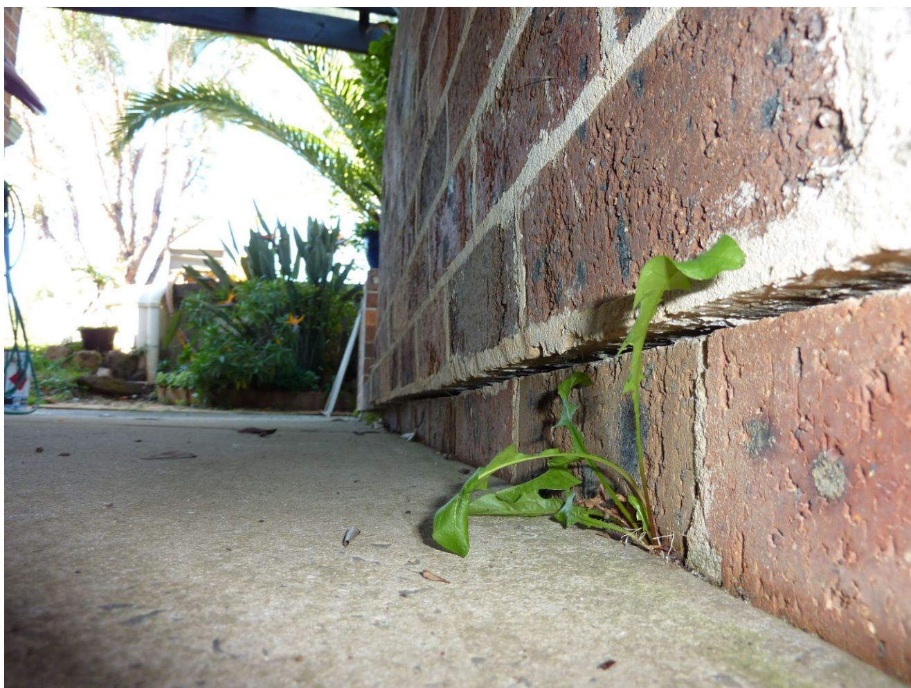
Figure 9 – Mine subsidence resulted in damage along a mortar bed where an external pavement was formed against an external brick wall
