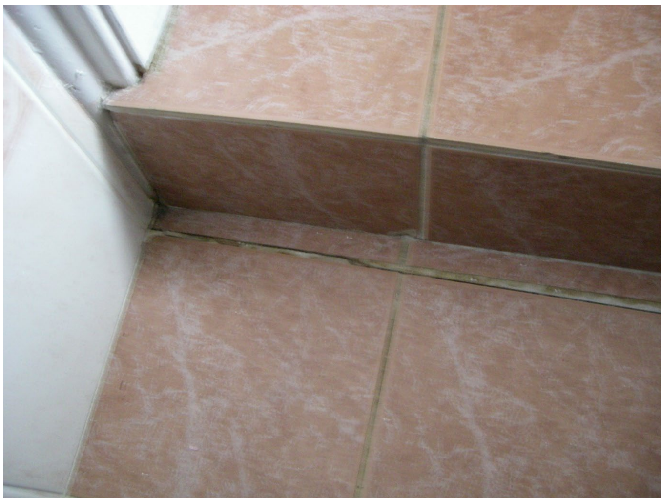
Figure 8 – Mine subsidence resulted in cracking of floor tiles directly aligned with the same step in ground slab shown in Figure 4.
