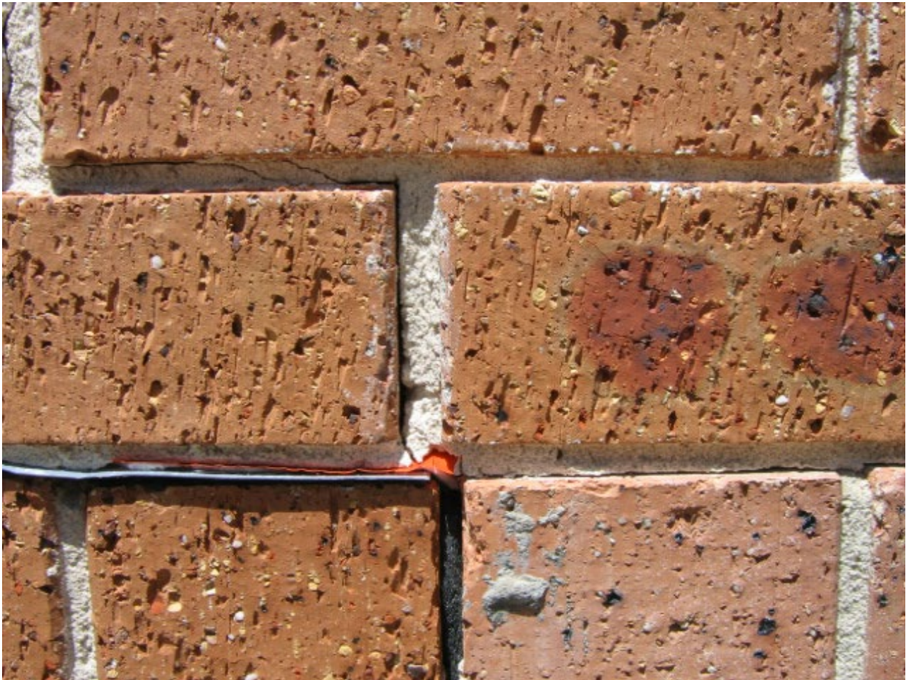
Figure 5 – Mine subsidence resulted in a crack that concentrated at a step in the damp proof course
