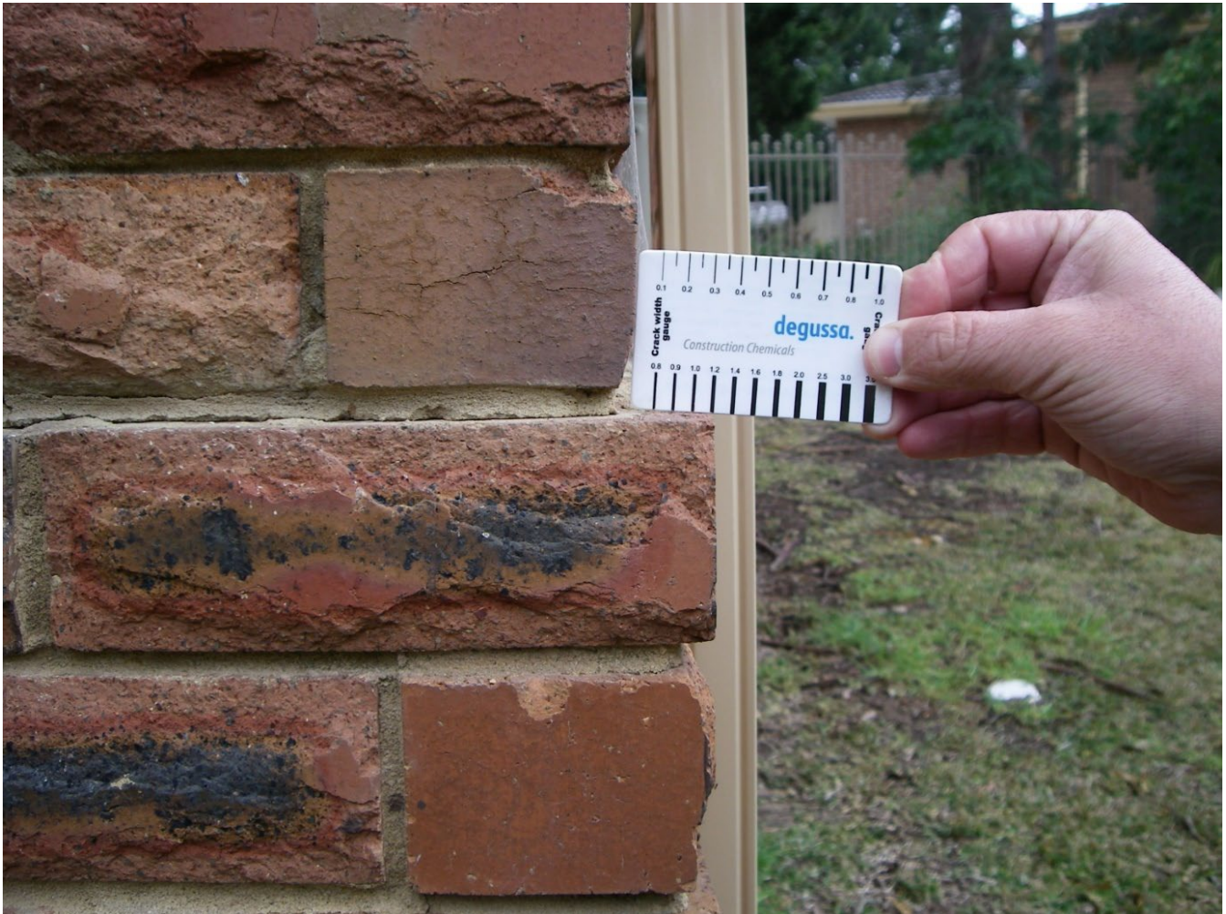
Figure 6 – Mine subsidence resulted in slippage of the damp proof course (this is an extreme example)
