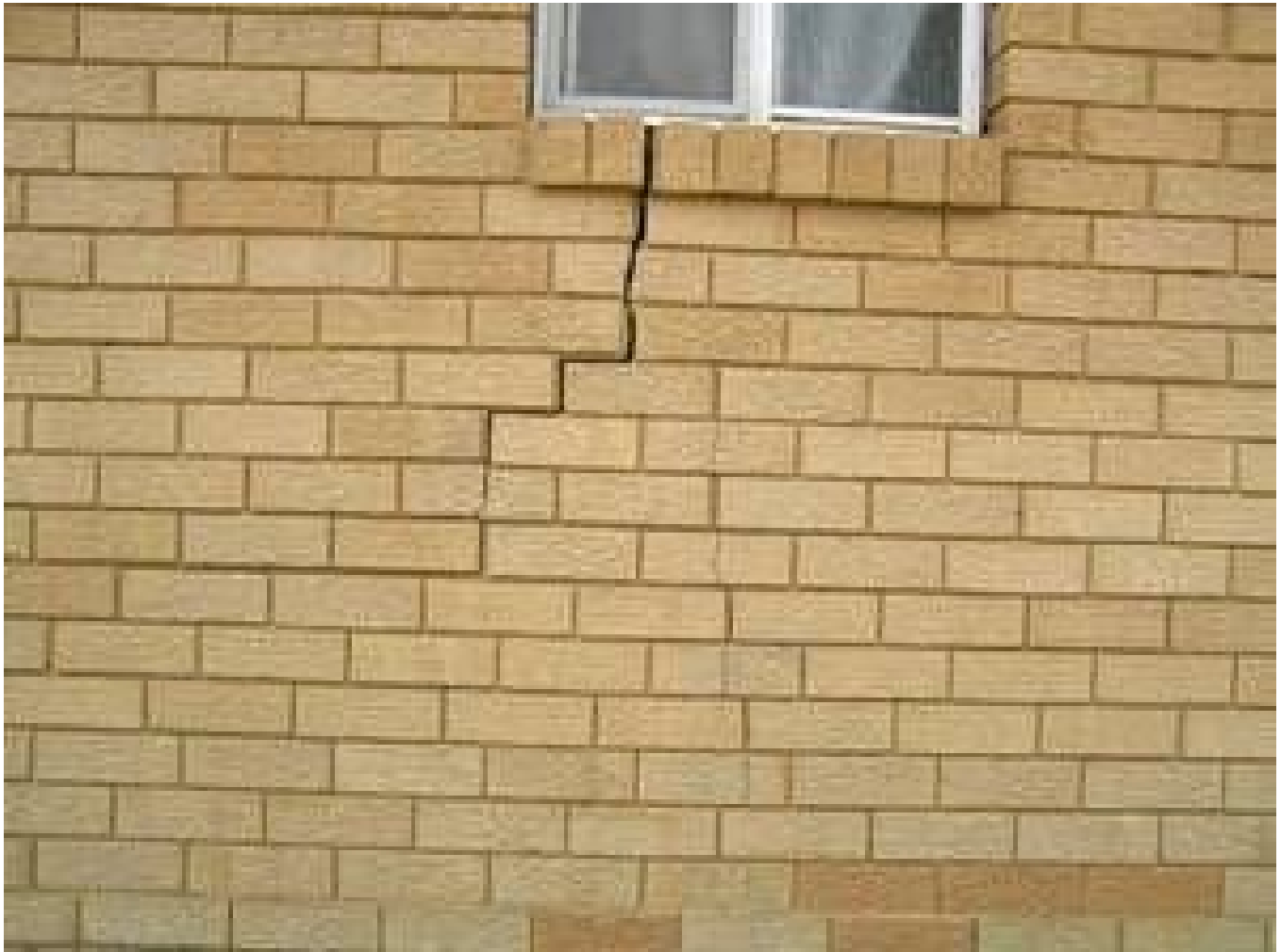
Figure 7 – Mine subsidence resulted in cracking around window openings (this is an extreme example)
