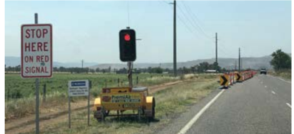
Temporary traffic lights on a road. You must stop on a red signal.
