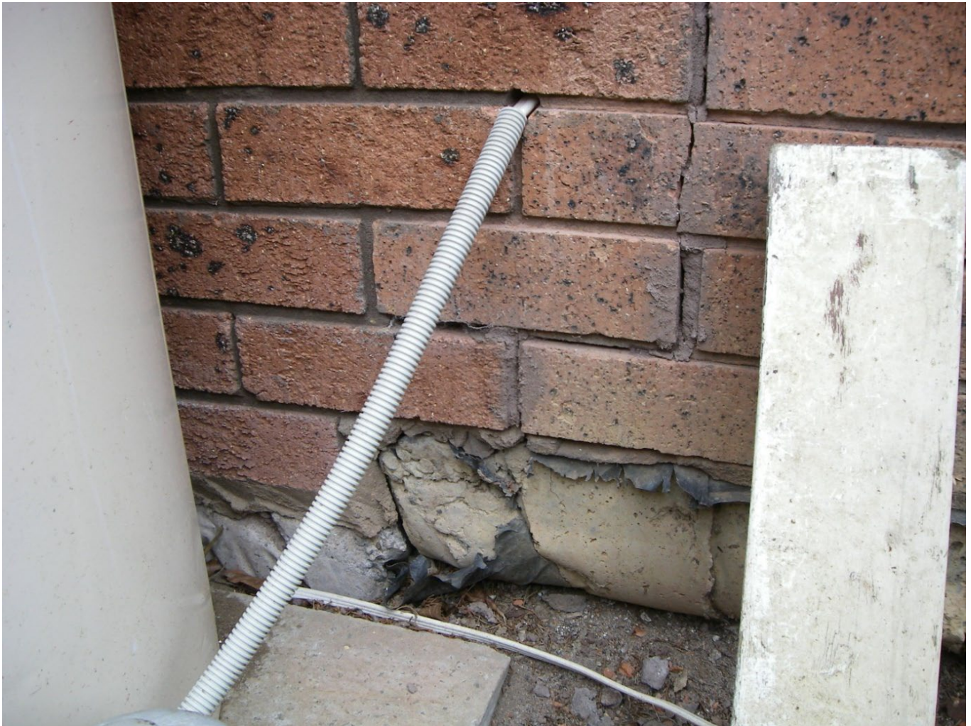
Figure 3 – Mine subsidence resulted in a crack, which has occurred between two separate ground slabs that are founded at different elevations, with no articulation joint in the overlying brickwork.
