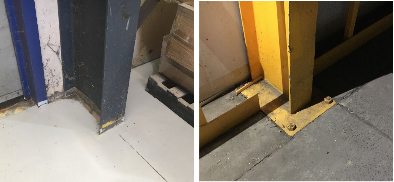
Figure 4 – Column baseplates are recommended to be exposed to facilitate future inspections and adjustment if required
